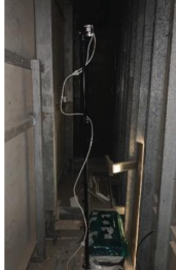
Entire Sealing Station Inside Exterior Wall Cavity
