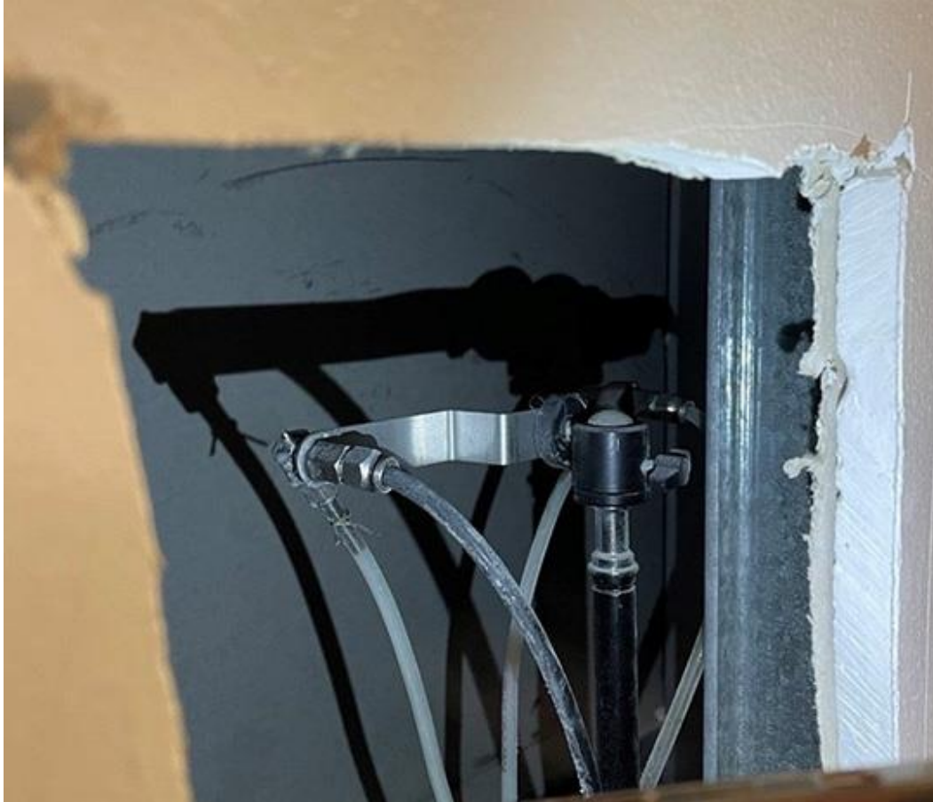
Sealing Station Spray Nozzles Inside Exterior Wall Cavity
